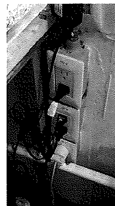
Tomacorrientes dúplex. Volts. 127 volts.
